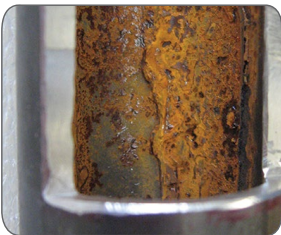
Atmospheric dirt Rust or corrosion Deposits from pipe walls
